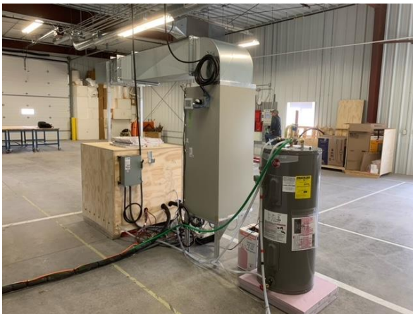
Figure 12: Compressor box, indoor air handler and a 50-gallon water tank
