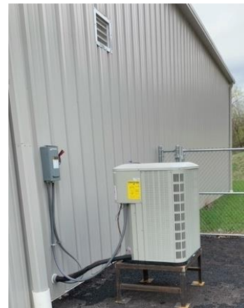
Figure 13: outdoor unit containing a fan and a microchannel coil
